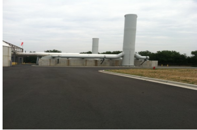
CCMUA's new Biofilter System
