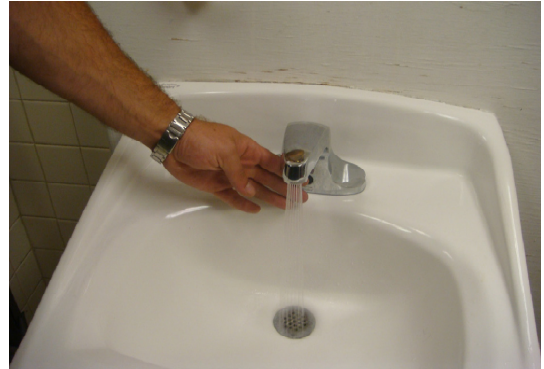
Install a high efficiency faucet aerator
